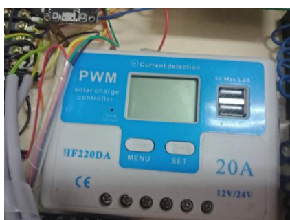
Solar Charge Controller
